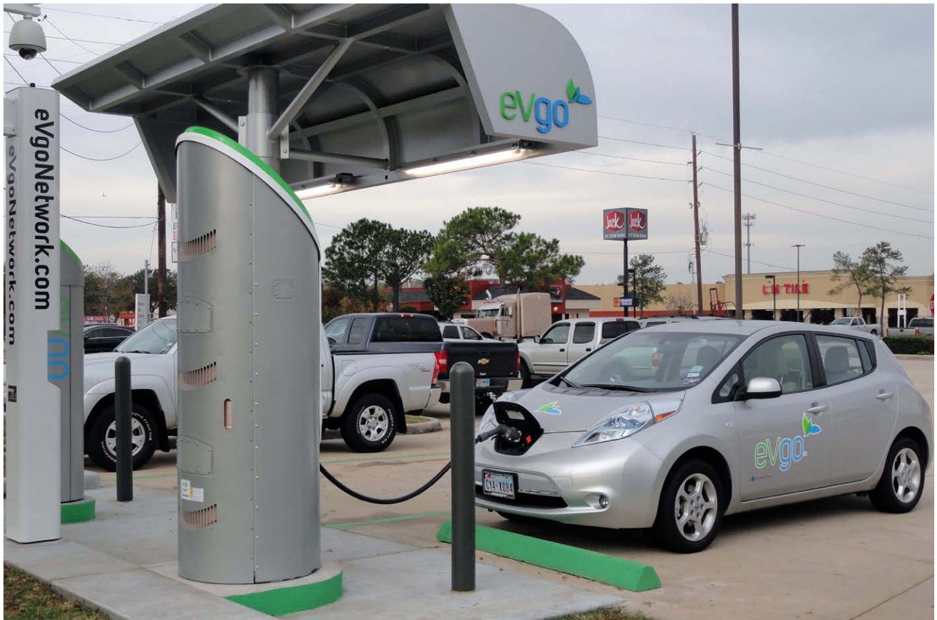
Electric vehicle charging stations
