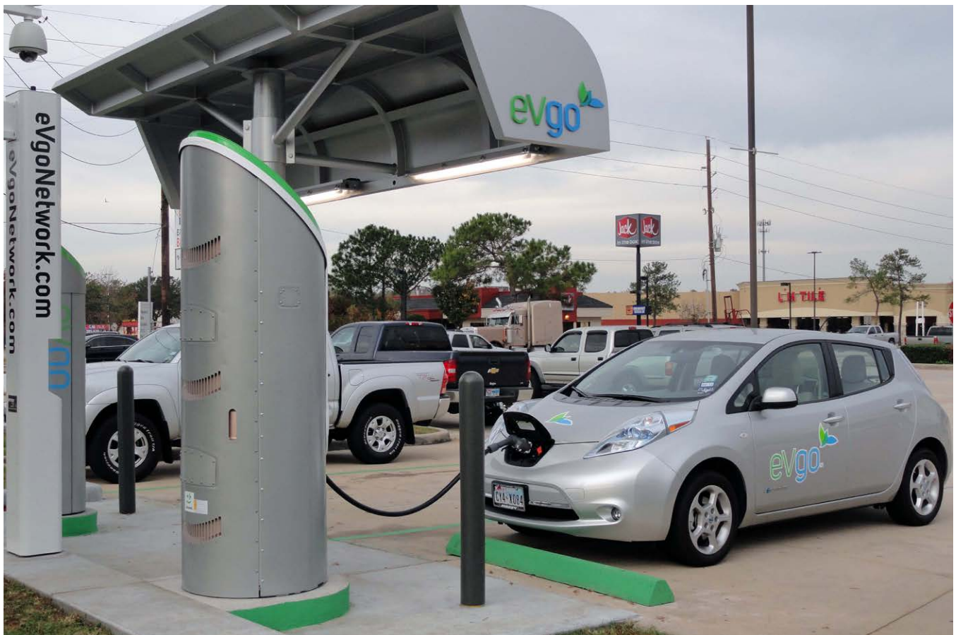
Electric vehicle charging stations
