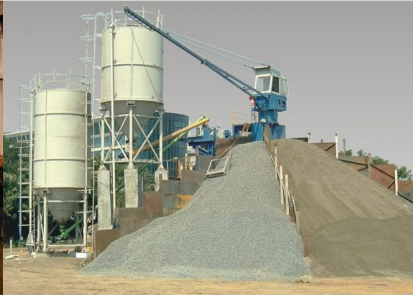
Concrete batch plants
