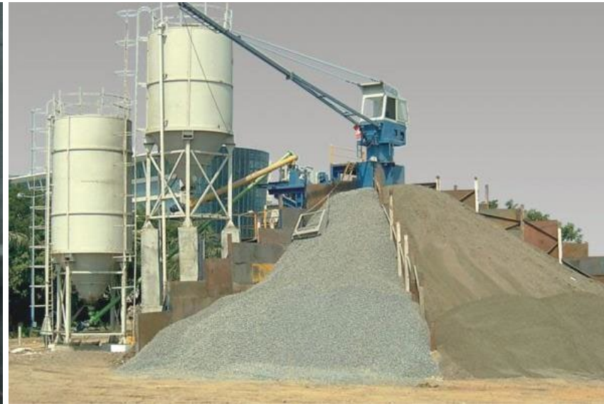
Concrete batch plants
